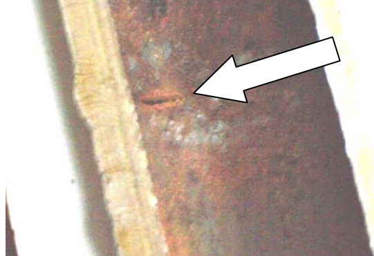
Photo 2- Failed portion from inside
